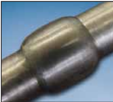
Connection between two Aluminum cables
