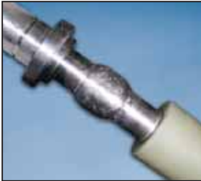
Terminations: Copper 'Top Bolt' on Aluminum solid cable
